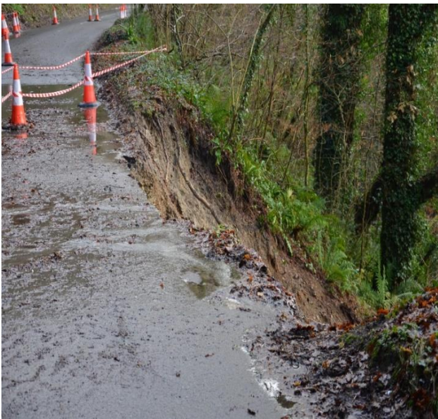
One of the slips causing the road closure Margaret Burgess
